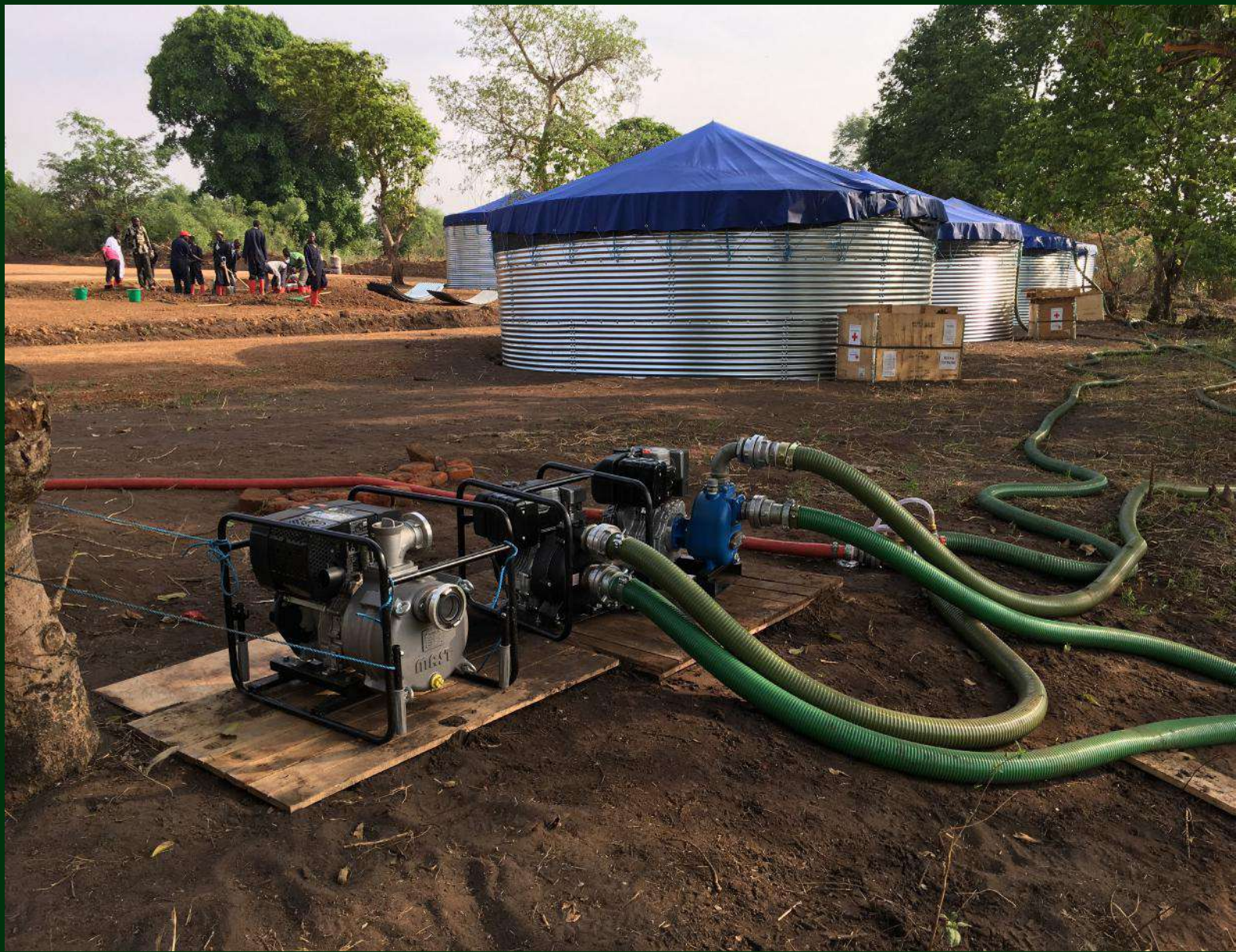
M40 Mass Sanitation Module Installation (Donated by Swedish Red Cross / Supplied by Butyl Products Ltd.) Uganda, 2017
